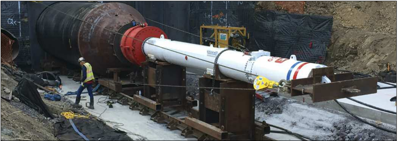
Figure 6. Tensioning System, Ryan Creek Project
