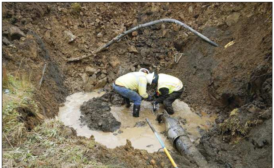
Unknown crossing utility damaged during excavation, not the pipe bursting process
