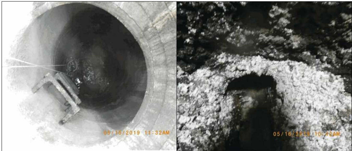
This manhole looks good from above, but closer inspection uncovers problems.
