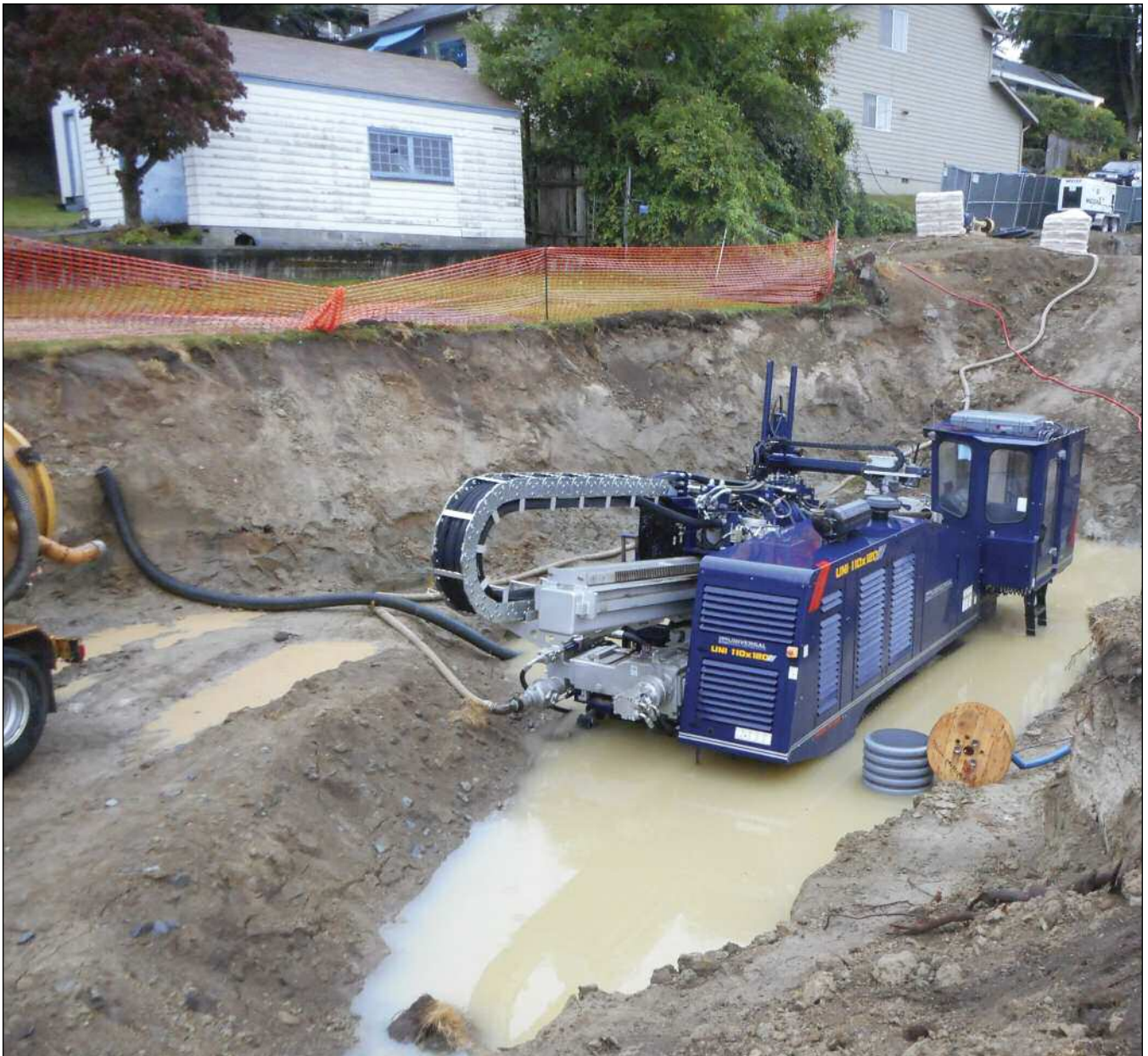
Equipment became flooded with water at one point in the Talbot Hill project.
