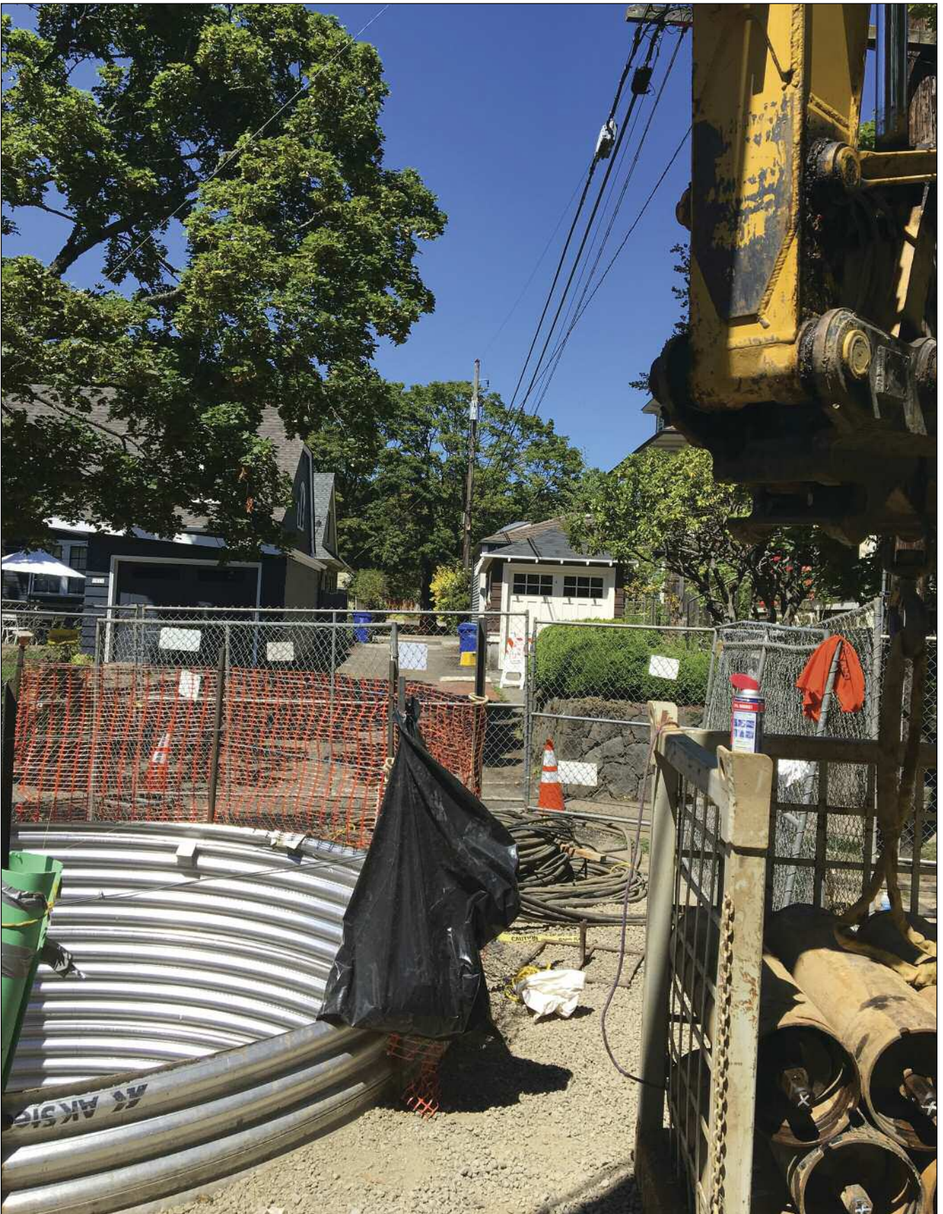
A 9-foot shaft made trenchless installation in this tight Portland alleyway practical.
