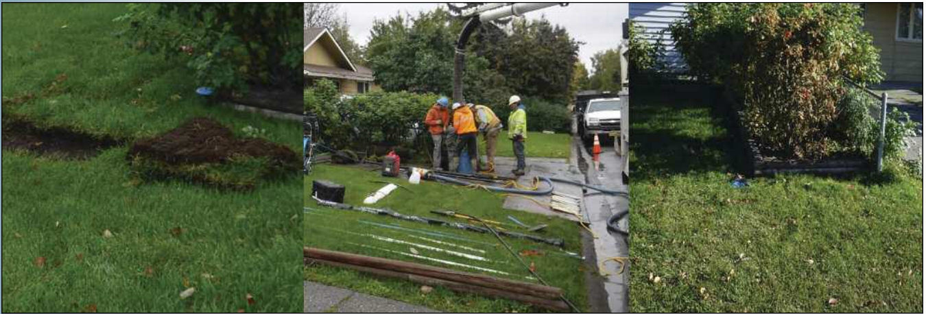
Steps in replacing a key box: preparation, including removal of strips of turf; crew's work on the key box; job completed, turf replaced.
