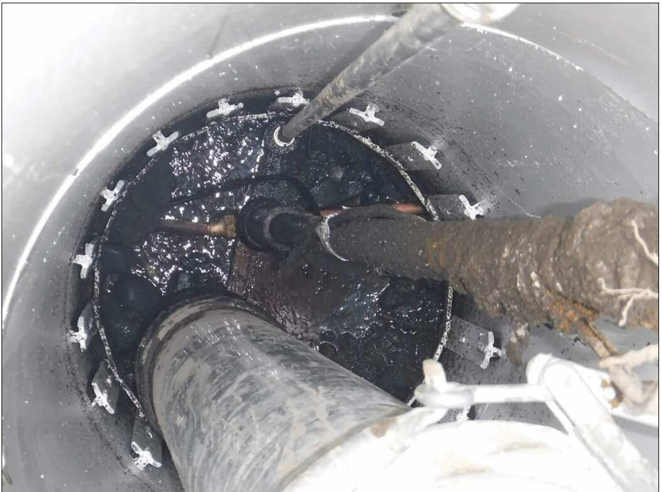
AWWU decided to build on the experience of a Canadian city to develop a process for removal and replacement of key boxes.
