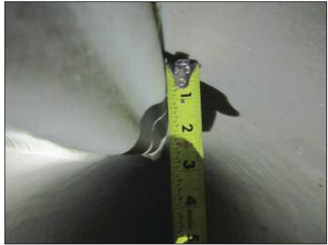
Figure 3. Severe WFF in poorly handled liner
