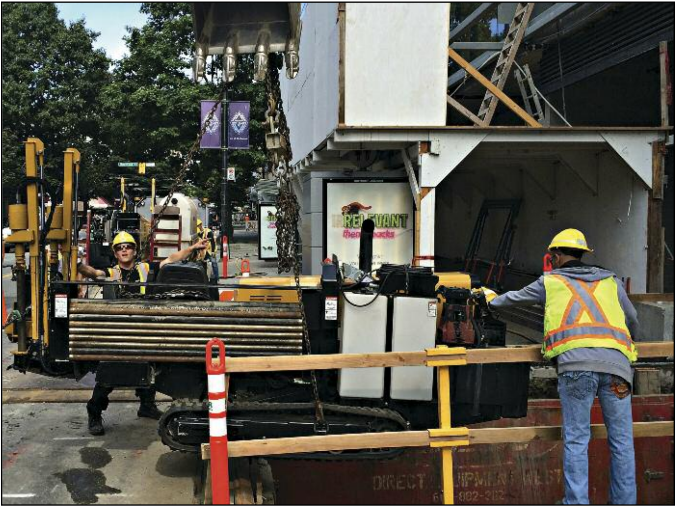
The Canadian City of Vancouver added trenchless technologies to its sewer operations construction toolbox in 2015.
