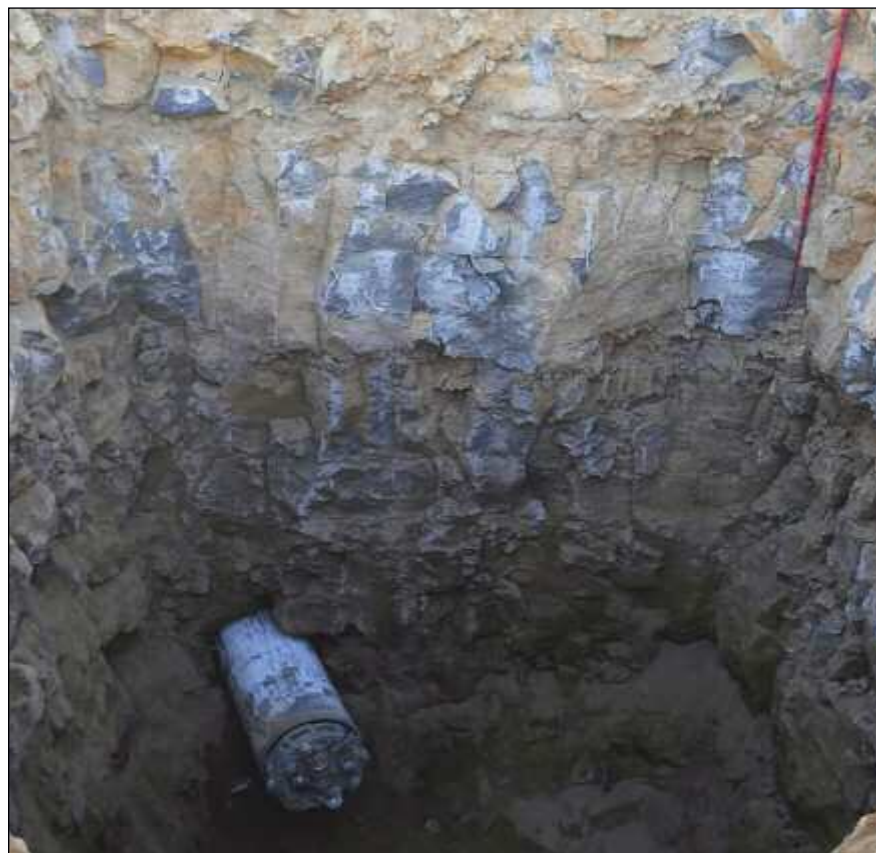
The Robbins SBU-RC broke through two weeks ahead of schedule on May 5, 2015. The blocky basalt subsurface conditions are seen here at the exit pit.
