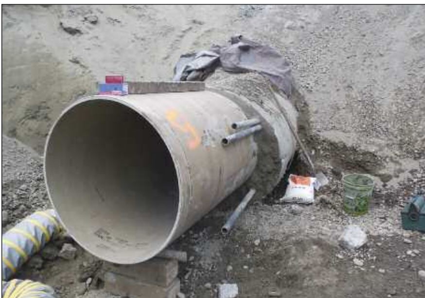
Annular space grout strengthened the system and filled voids in the host pipe.
