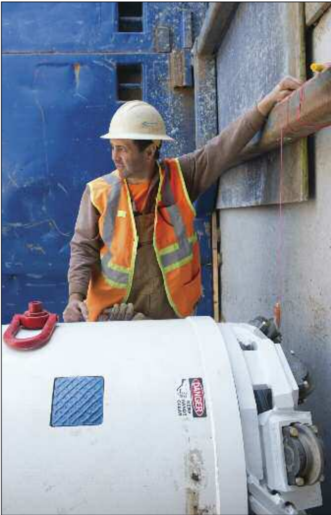
The Stadeli crew lines up the SBU-RC in the launch pit to bore a 323-foot-long crossing for a new gravity sewer interceptor.
