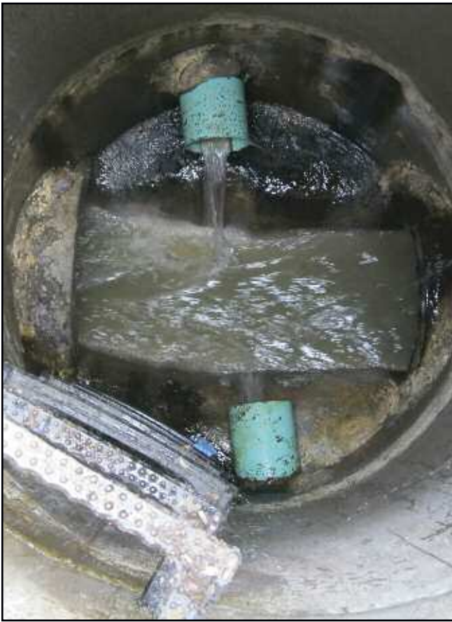
Figure D: Manhole condition prior to rehab
