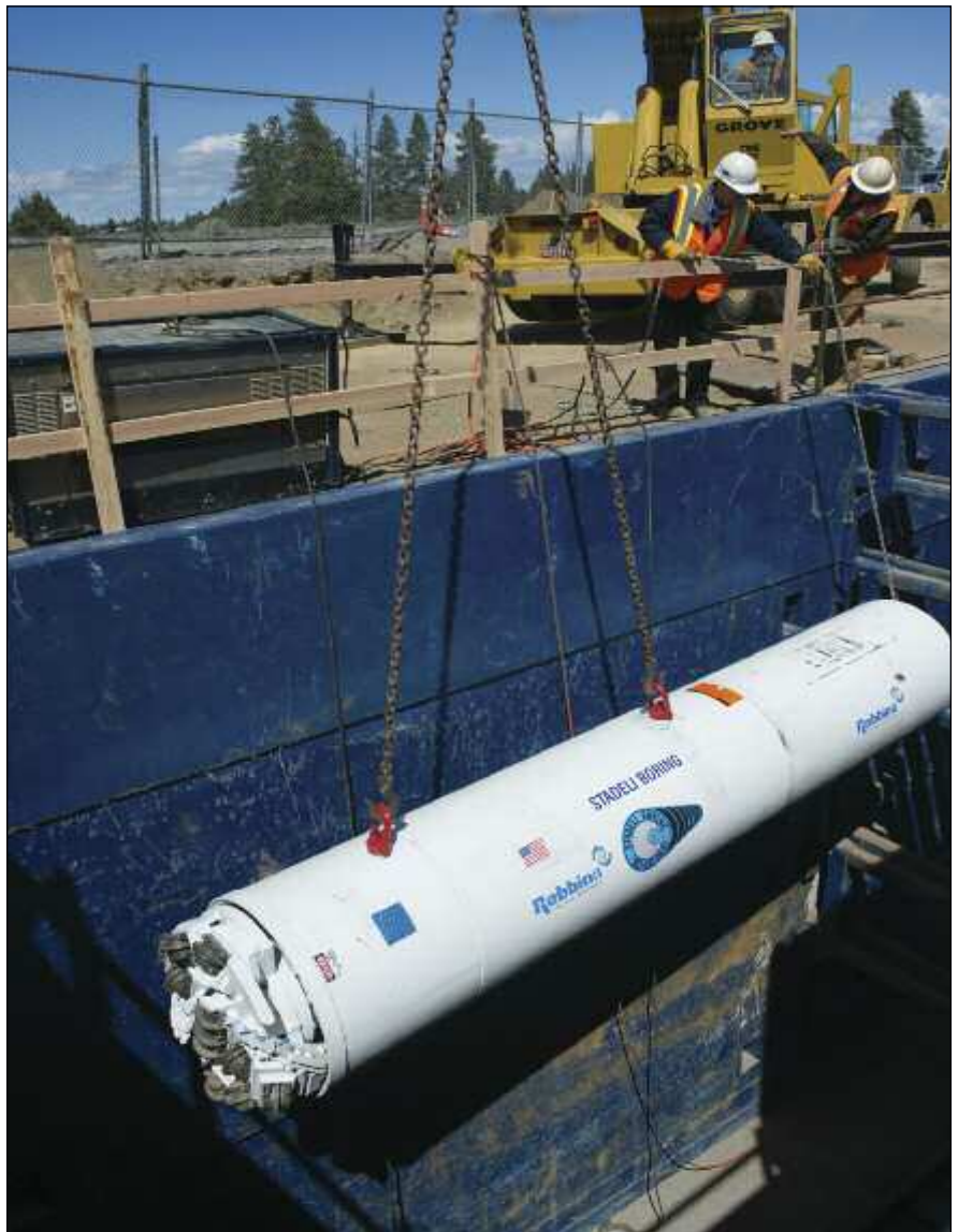
The Robbins 36-inch-diameter SBU-RC was launched at a jobsite in Bend, Oregon, for contractor Stadel Boring & Tunneling in April 2015.
