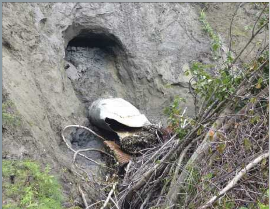
Collapsed outfall pipe and slope failure
