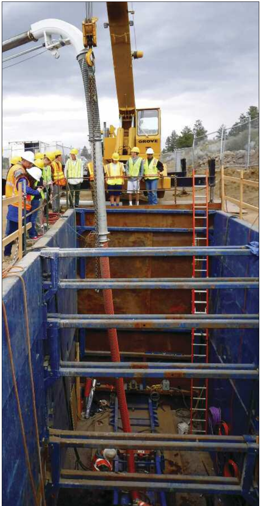
Spoils are removed from behind the SBU-RC cutterhead directly to the surface using a vacuum truck.
