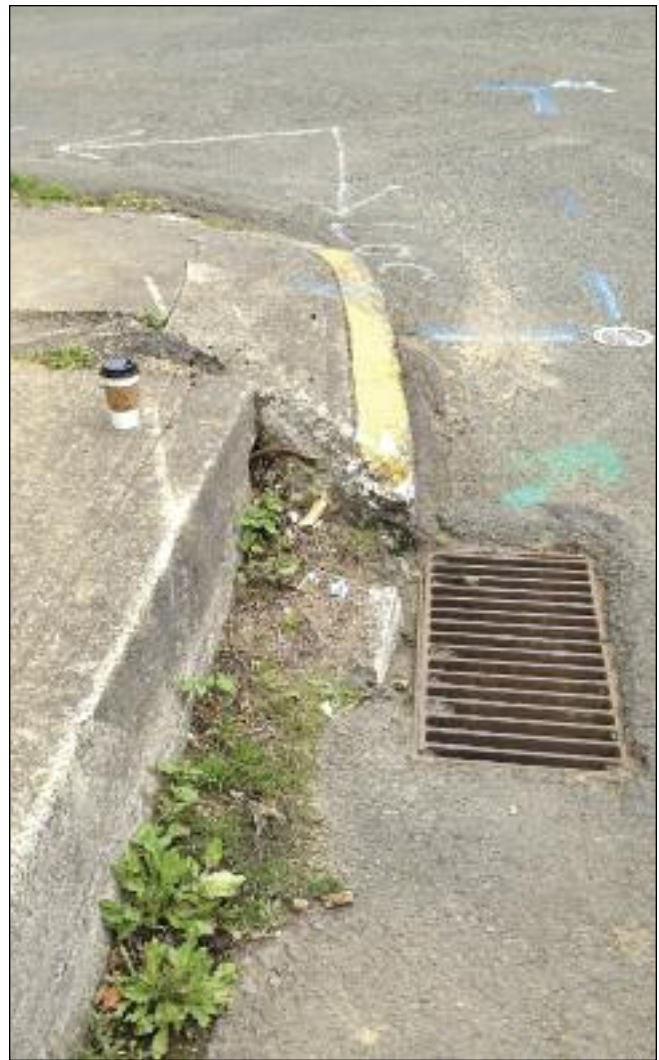
Creeping earth movements crack pavements and other infrastructure in Astoria.
