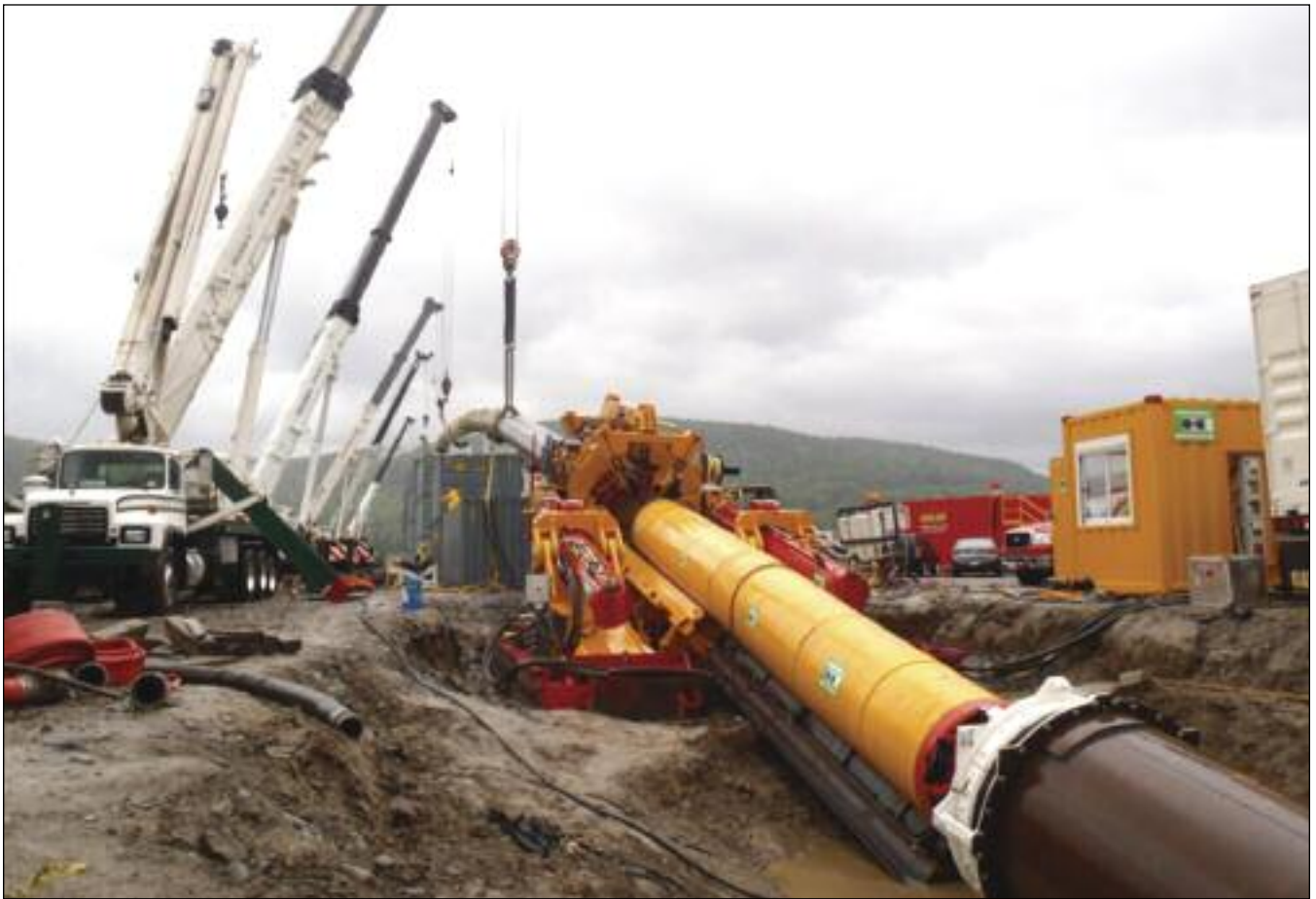
Figure 2. Installation of a 42-inch steel pipe in New York, August 2011. Photo provided by Herrenknecht AG.
