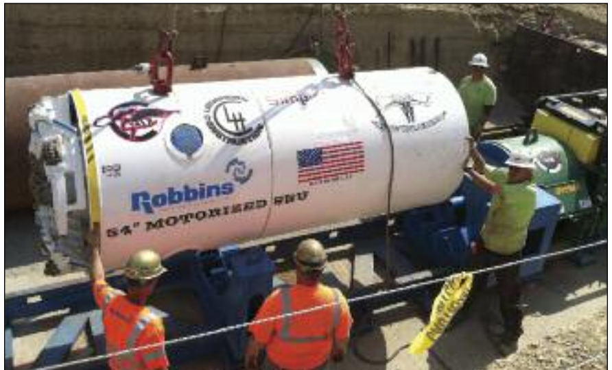
A 54 inch (1.4 m) diameter Robbins Motorized Small Boring Unit (SBU-M) was used on two mixed ground bores in Wyoming, USA
