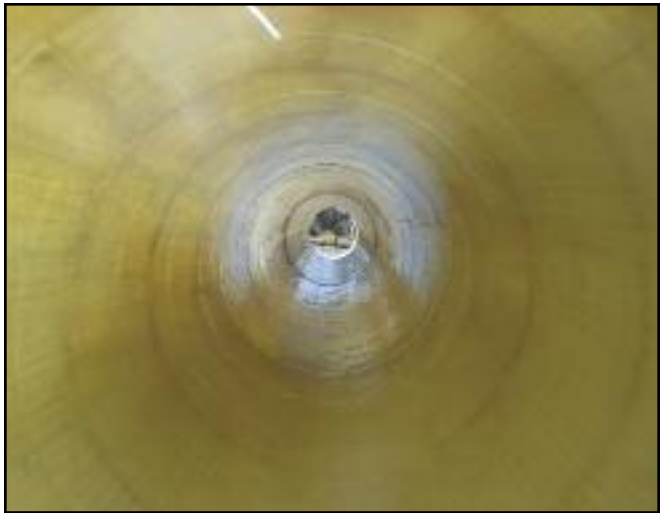
Figure 4. StifPipe at Arc Terminal – completed installation
