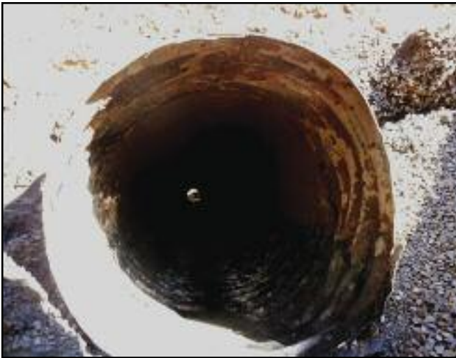
Figure 3. Highly corroded culvert at Arc Terminal
