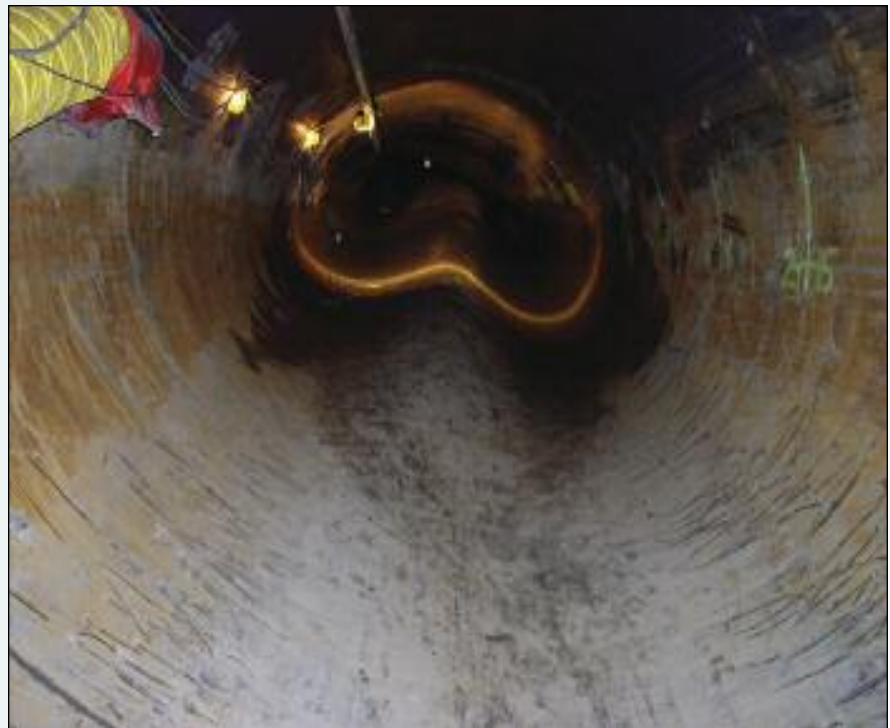
Figure 1. Deformation of Pipe
