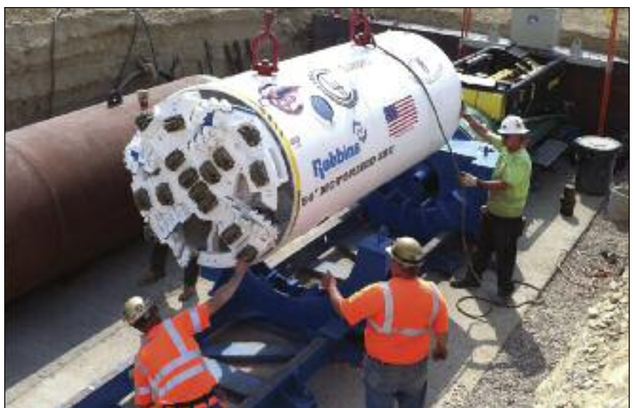
Robbins Field Service personnel were onsite to assist the contractor, Claude H. Nix Construction, in launching the Small Boring Unit
