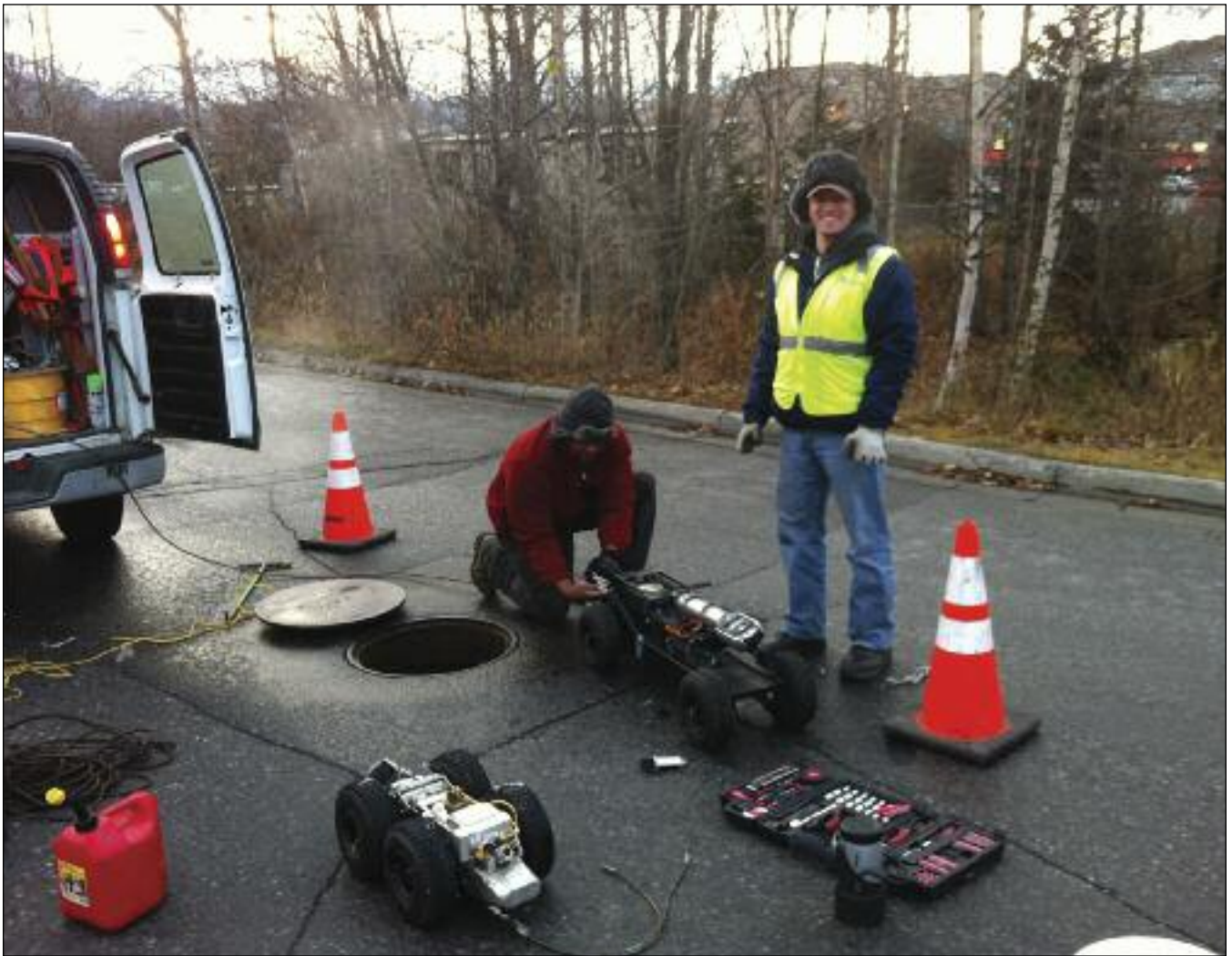
AWWU's sewer asset management plan is one tool in managing the risk associated with an aging sewer pipe system.
