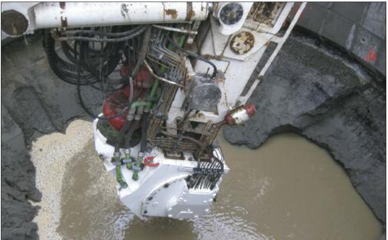
The Herrenknecht VSM is set into the shaft at the Ballard project's south site.
