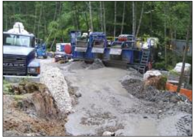
Excess mud flows out of the spoils pit
