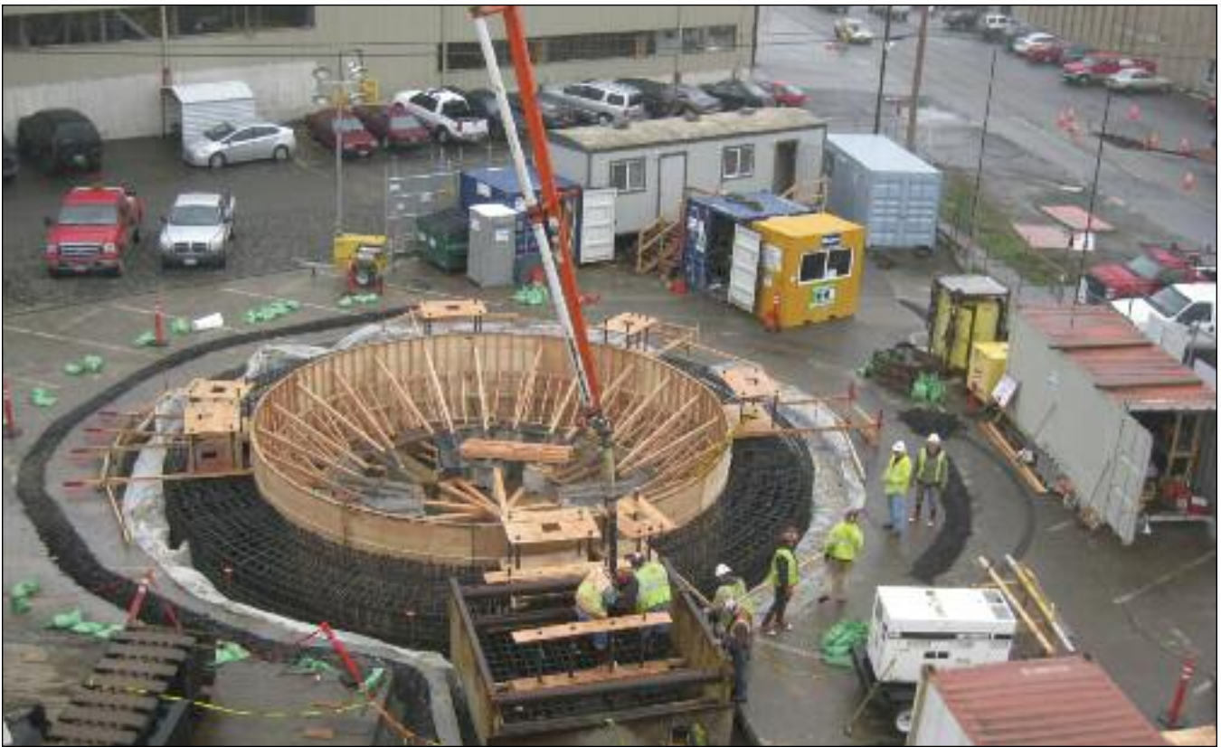
A guide wall for the Herrenknecht VSM is prepared at the Ballard project's south site.
