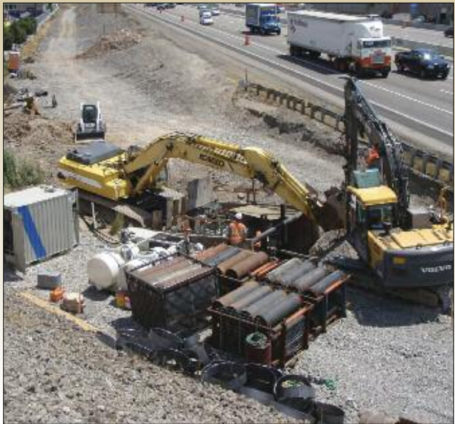
Minger Construction jacked 18- to 72-inch ID pipes with a guided boring machine system and several tunnel boring machines.
