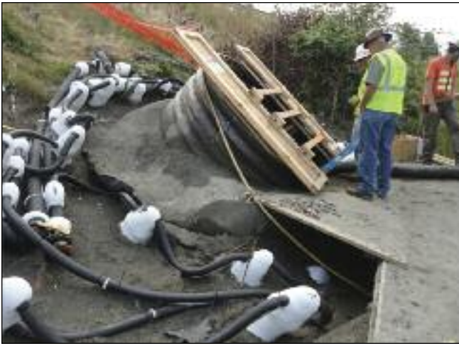
A concrete portal with steel liner plates was constructed and put into place.
