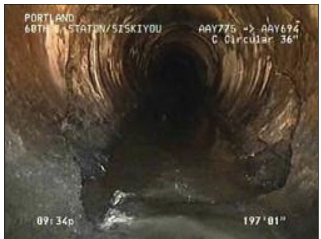
Existing deteriorated 36-inch sewer pipe
