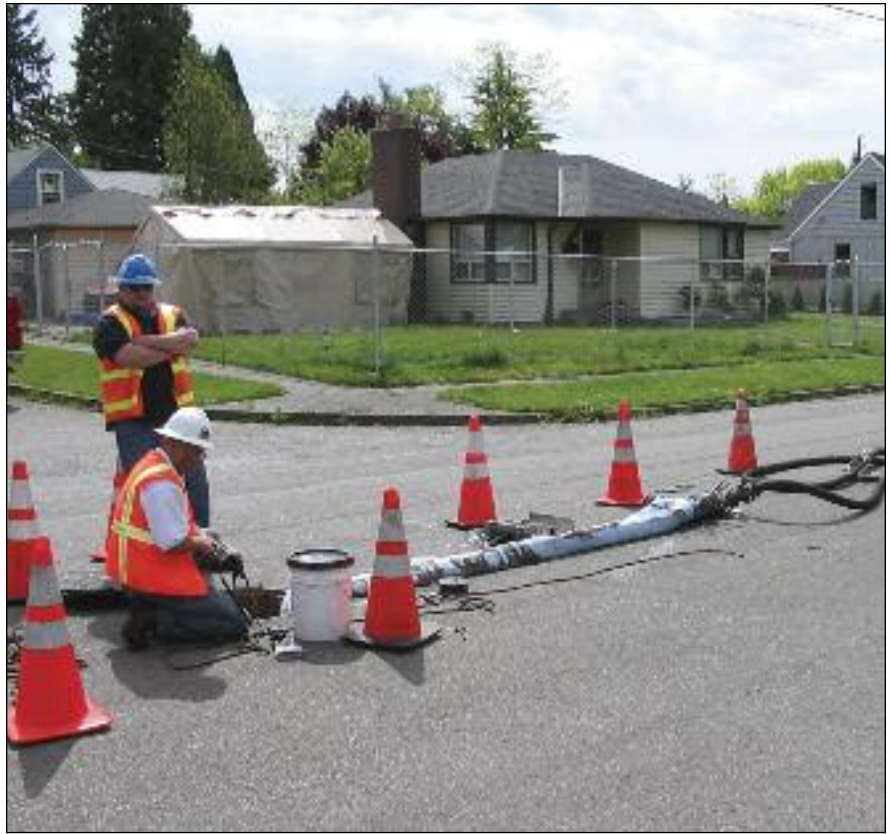
Rehabilitation of more than 63,400 feet of sewer lines was achieved at a total cost of less than $3.5 million.
