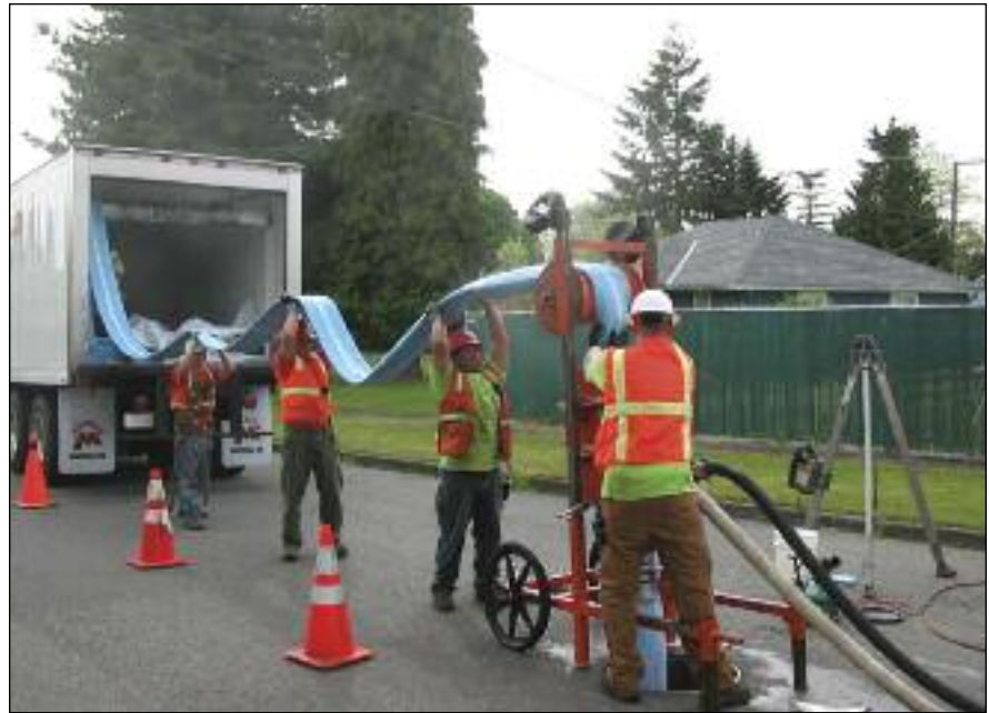
Liner installation (above) and open-cut repair for the Chelsea Park sewer rehabilitation project were split into two separate contracts.
