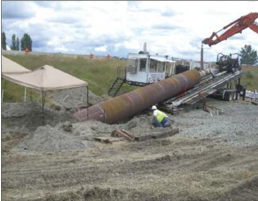
A 240-foot-long conductor casing was installed as part of Segment 5N of the Tulalip project.
