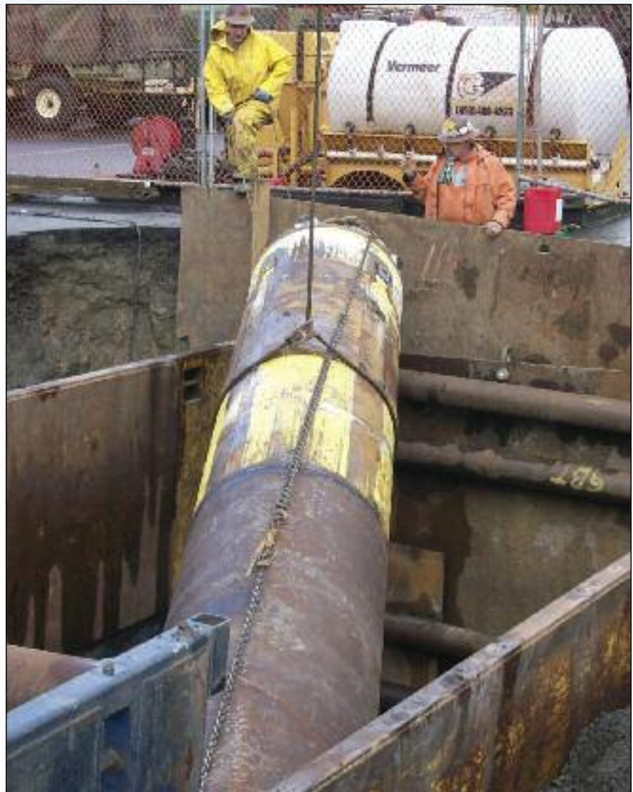
Gonzales Boring & Tunneling completed a new distance record using a Robbins Small Boring Unit.
