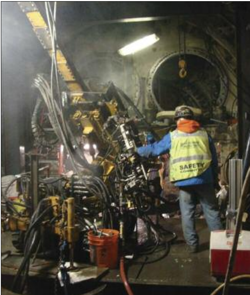
Angled freeze pipes below the bottom of the TBM were installed in drill holes using a small drill rig inside the TBM shell.
