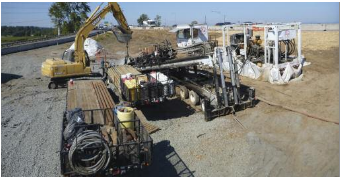
An American Augers DD-625 drill rig was used in Segment 5N of the Tulalip pipeline HDD project.
